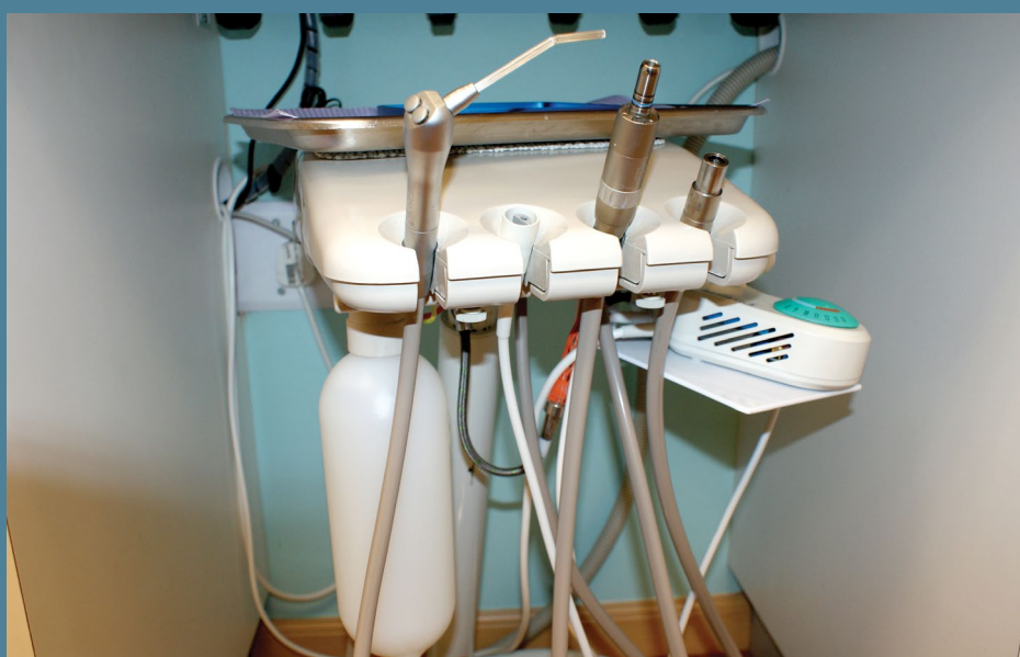
FIGURE 6.1: Narrow lumen of dental unit air- and waterlines
